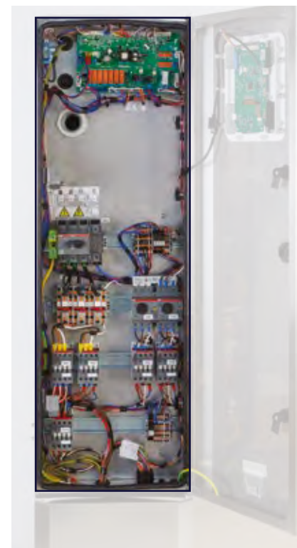
Single-point power connection
